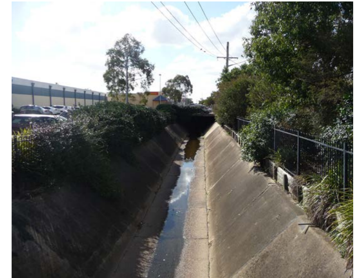
Figure 122: Exposed canal is unsightly.
