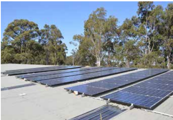
Solar panels installed at the Council Works Depot
