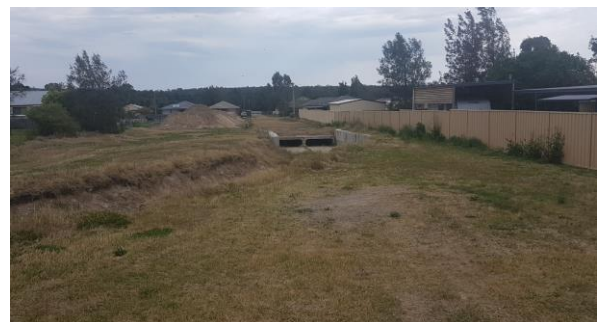
Photo 32: Culvert inlet (2m x 2.7m x 0.75m) installed between Kent St and Whitburn St
