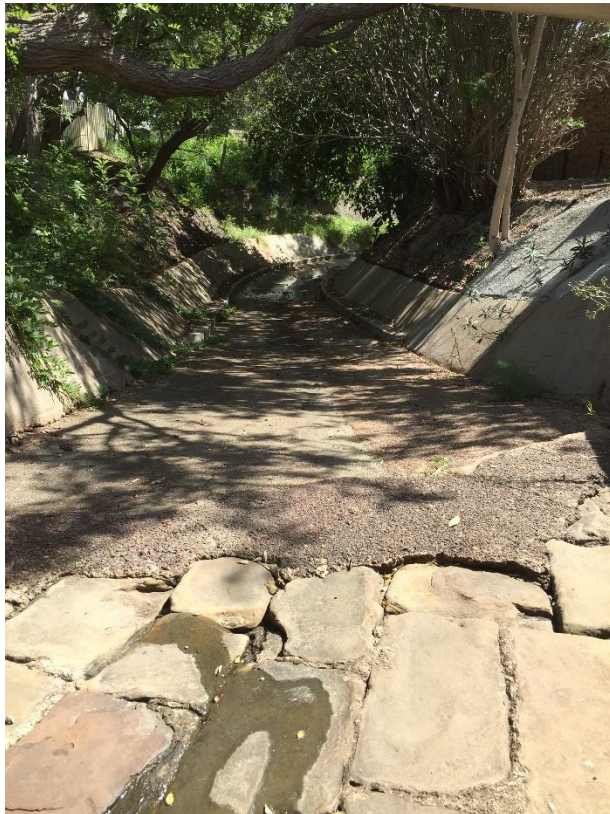
Photo 24: New England Highway – steep slope downstream of the hydraulic structure
