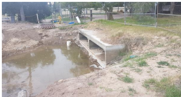
Photo 29: Culverts (2m x 2.7m x 0.9m) installed at the New England Highway
