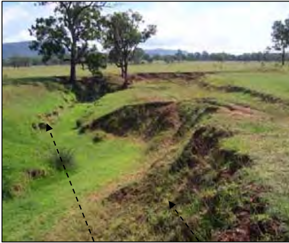
Limestone Creek channel showing significant bed lowering and bank erosion
