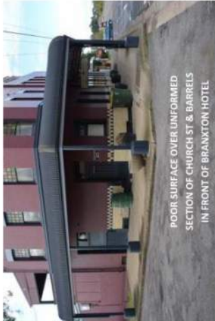
SOME ELEMENTS IN DISREPAIR AT CORNER OF CHURCH ST
