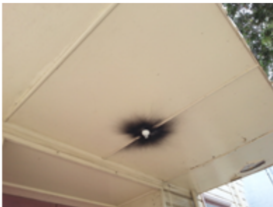
Deterioration in Building services
